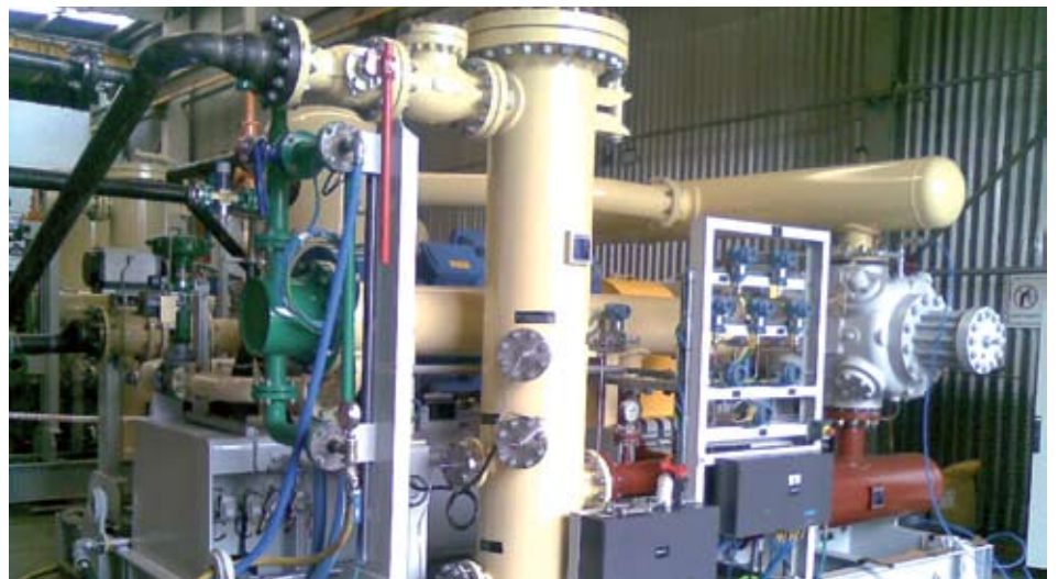
Flotech gas compression system being tested at the Auckland plant
