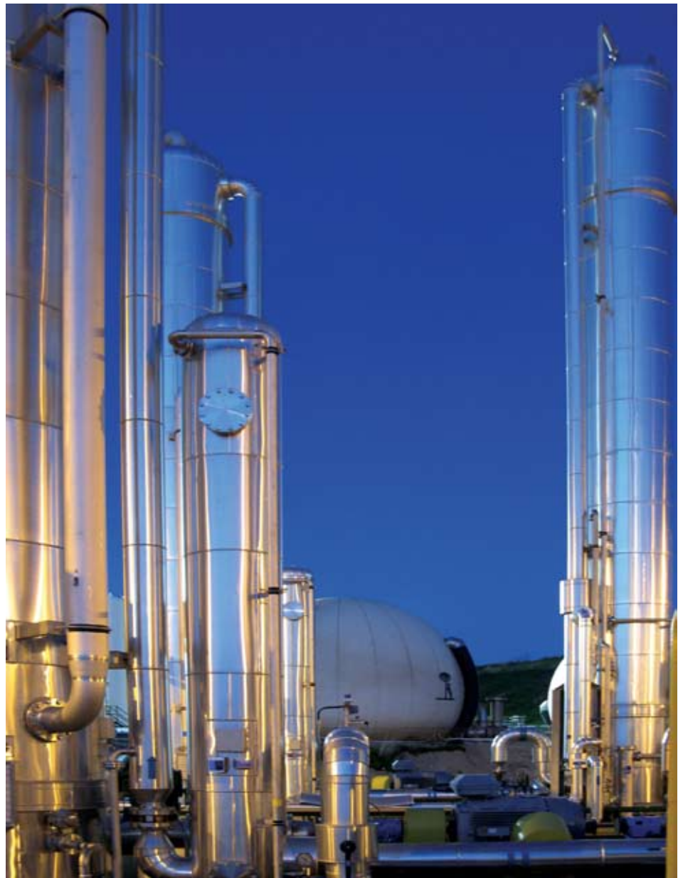
Madrid Biogas Plant
