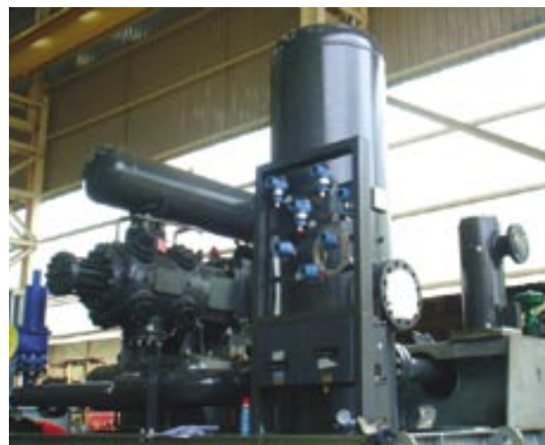
Kuwait Development Booster Compressor Package
